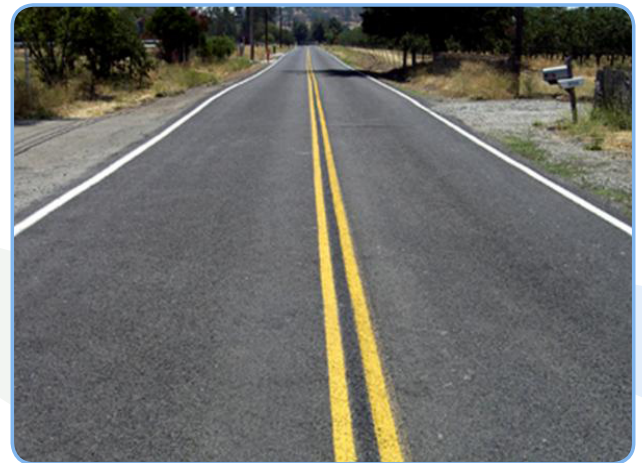
In 2005, status of a deforming road before Chip Seal application
