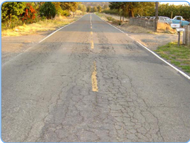
In 2005, status of a deforming road before Chip Seal application
